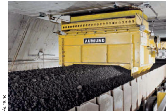
14 Clinker storage discharge
