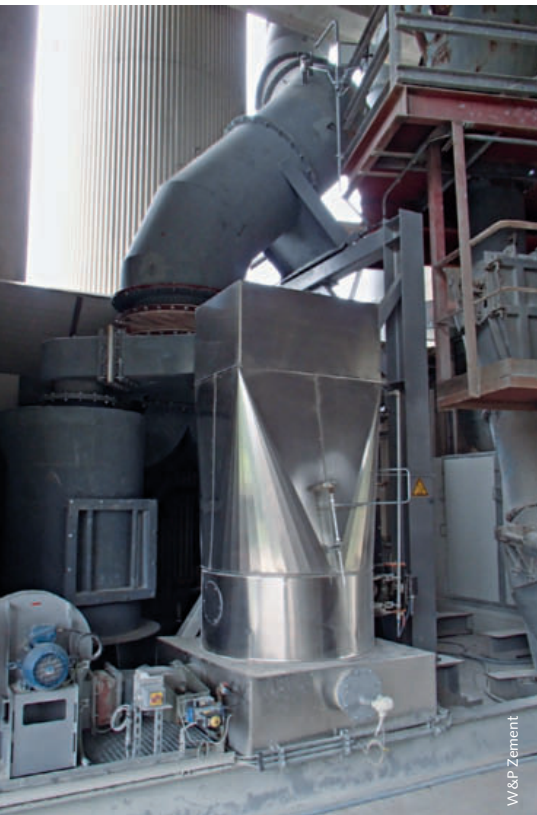
7 Partly visible cyclones for separation of the heated dust particles after the thermal treatment in the second preheater line
