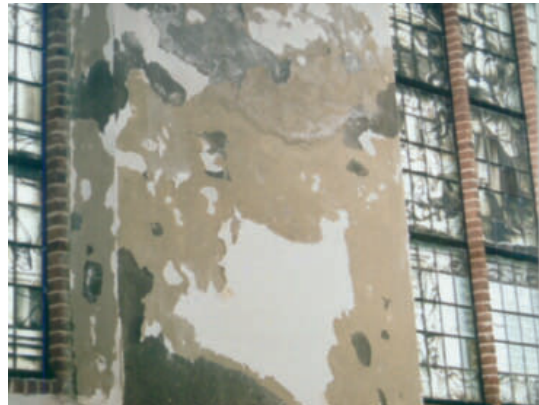
1 Salt damage in pointing mortar (left) and plaster (right)
